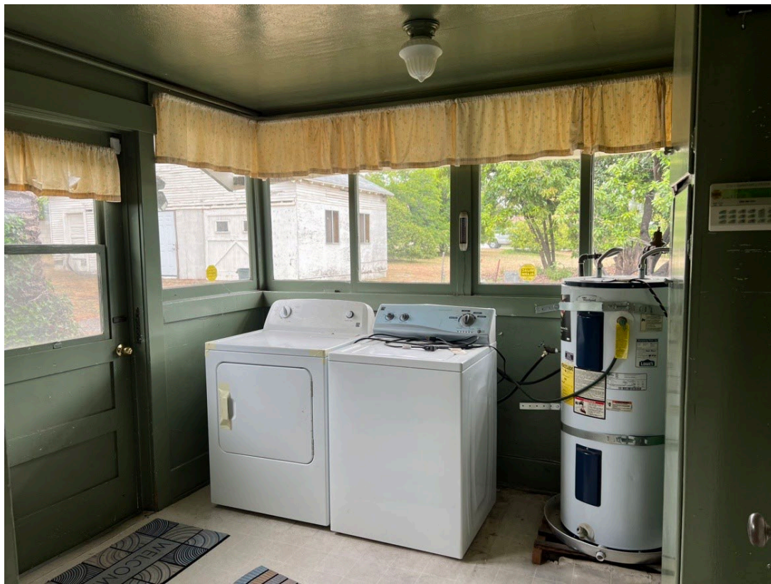
Figure 9. Main house utilities room
